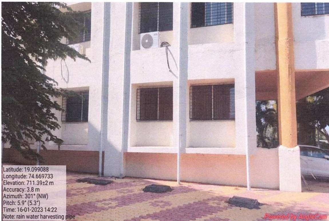
Image: Rain water collection pipe
