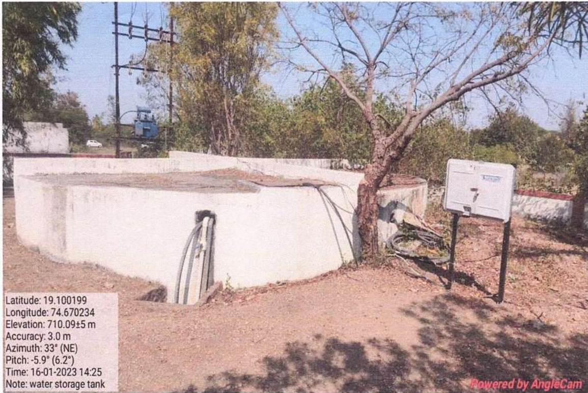
Image: Water storage tank
