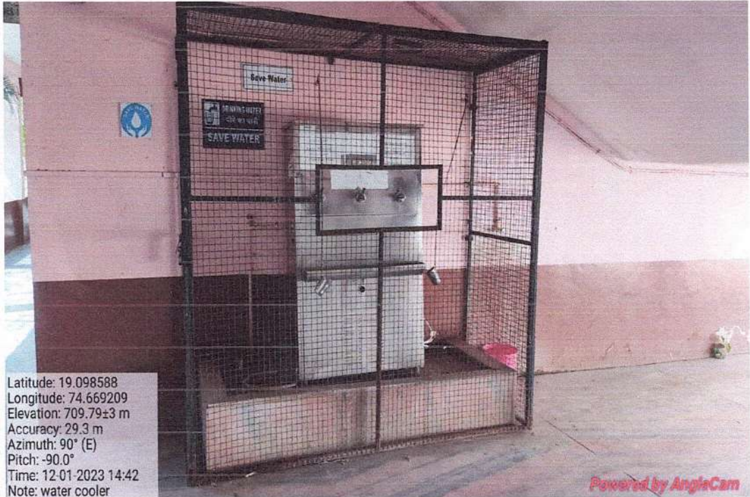
Image: Water Cooler
